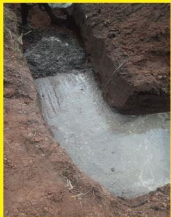
Casting of foundation for the ongoing fencing of ESN plot for National Secretariat at the University of Abuja
