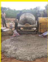
Casting of foundation for the ongoing fencing of ESN plot for National Secretariat at the University of Abuja
